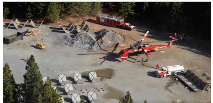
Contractor prepares to use a helicopter to fly in precast flume sections for placement
