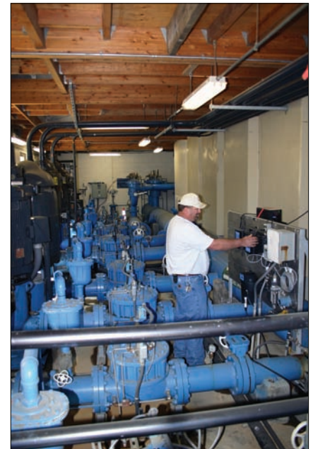
EID owns and operates five water treatment plants, two primary wastewater facilities, and four satellite sewage treatment facilities.
