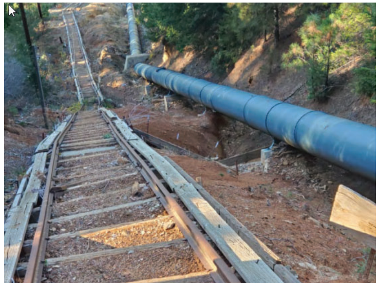
Erosion on Old Tram Way
