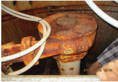
Corroded Filter Backwash Waste Valve
