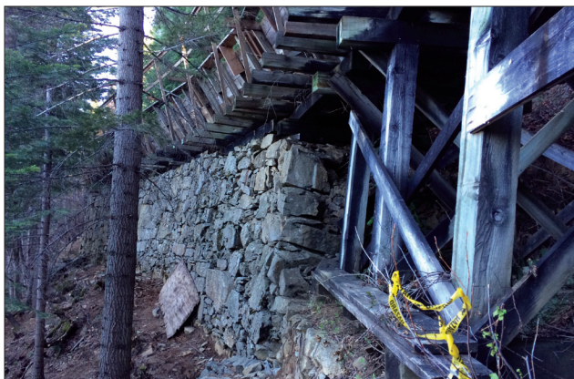
These pictures of Flume 48 show detail of the 139-year-old hand-stacked bench upon which the flume is built. The photo above shows the same cutout in the bench in 1923 that is shown in the 2015 picture below it.
