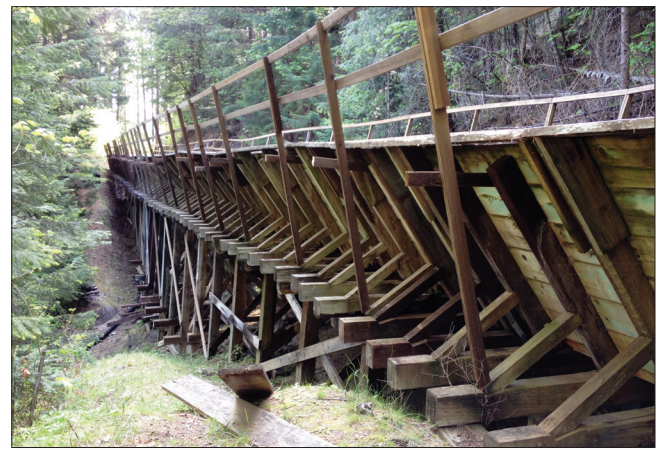
Flume 44, located directly above Highway 50, is a 67-year-old elevated wood flume that was last replaced in 1948. The flume traverses an active landslide that will be stabilized as part of its replacement.
